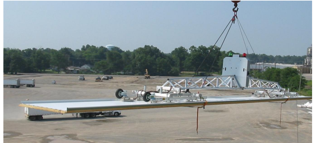
Pneumatic panel lifting equipment
