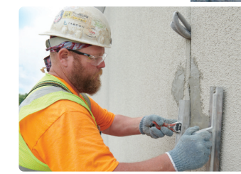
A stitch in time...timely maintenance and repairs can keep small problems from becoming big ones.
