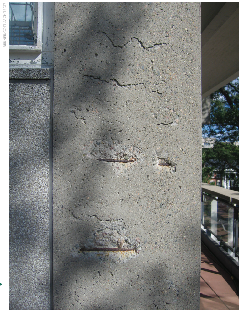
Exposed rebar or cut away concrete with rebars and anodes.
