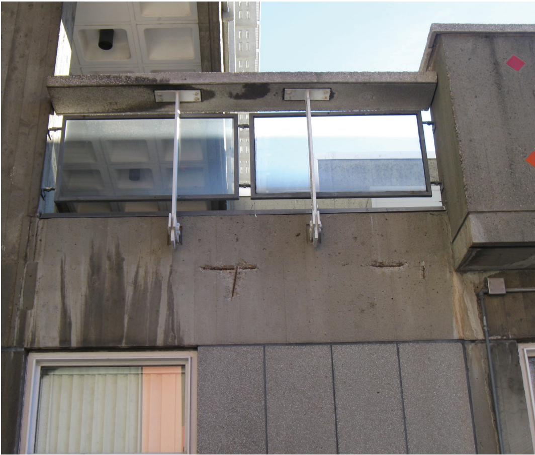
Five different surface treatments in one area of a concrete façade.
