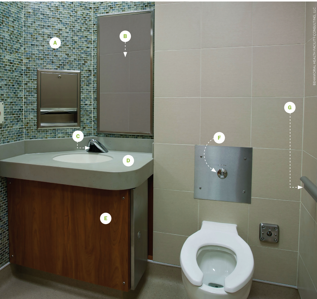
▲ Behavioral health patient bathroom with homelike wall and floor finishes (A); shatter-resistant mirror that will not produce loose shards when broken (B); ligature-resistant faucet (C); residential-style, ligature-resistant countertop-mounted sink with space for patient's toiletries (D); below-sink enclosure (E) conceals plumbing and houses bedpan washer behind the stainless steel door—special tool required to open door; ligature-resistant recessed push-button flush valve (F); and ligature-resistant grab bar (G).
